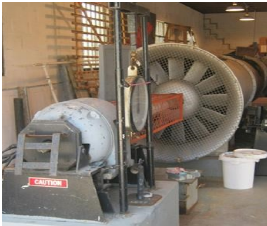
Figure 3.4 Missouri S&T surface main fan
