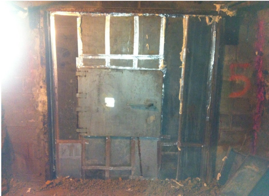
Figure 3.16 Kennedy steel door
