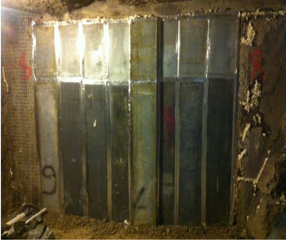
Figure 3.15 Kennedy steel stoppings as installed in the mine
