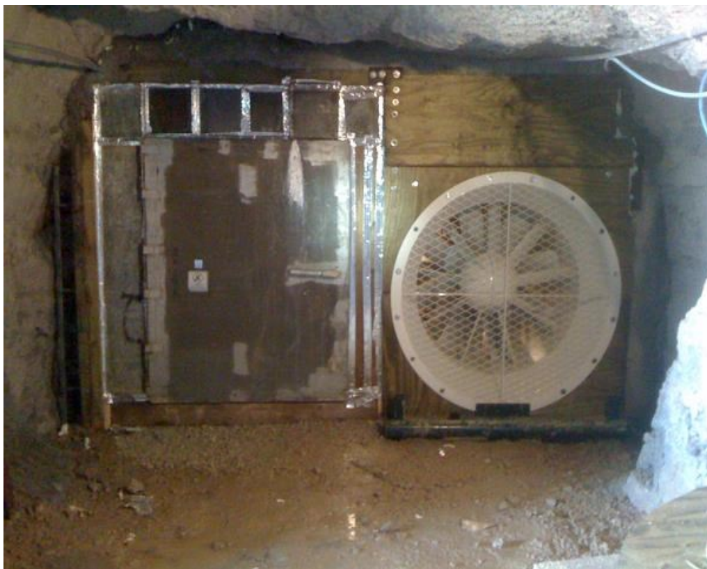
Figure 3.11 Booster fan bulkhead- rear view
